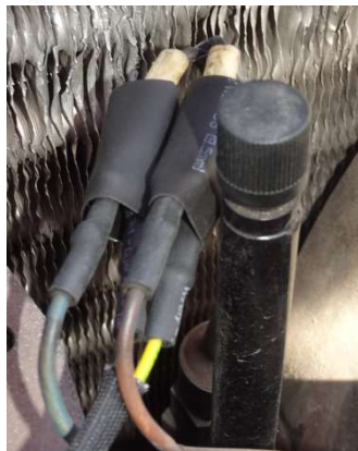
Additional two connections at the Temperature Switch Refrigerant
